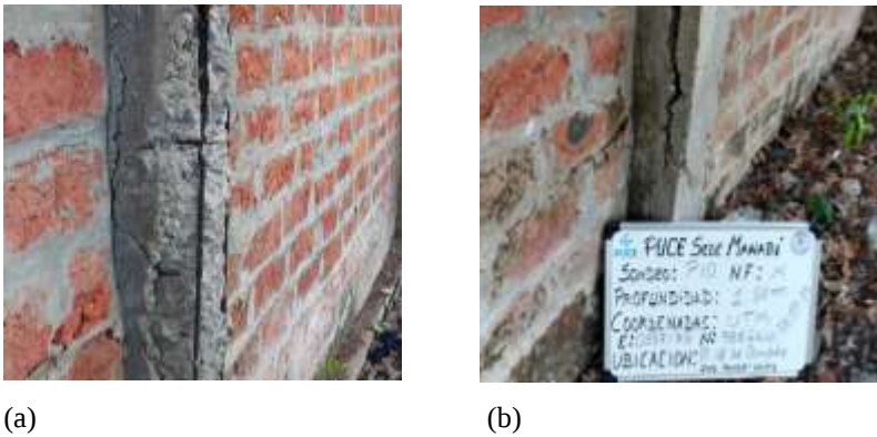
Figure 3. (a) Corrosion of reinforcing steel in a perimeter column near borehole P-10 due to very severe sulfate conditions in the soil. (b) Cracking and steel corrosion in another column of the same perimeter wall.
