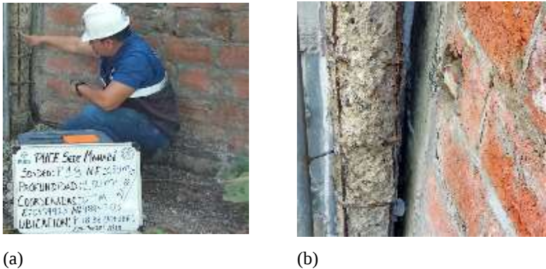
Figure 11. (a) Reinforcement corrosion in borehole P-18, with a groundwater table at 1.5 m depth. (b) Deteriorated concrete column with exposed and corroded steel reinforcement due to severe sulfate conditions, observed at borehole P-18.
